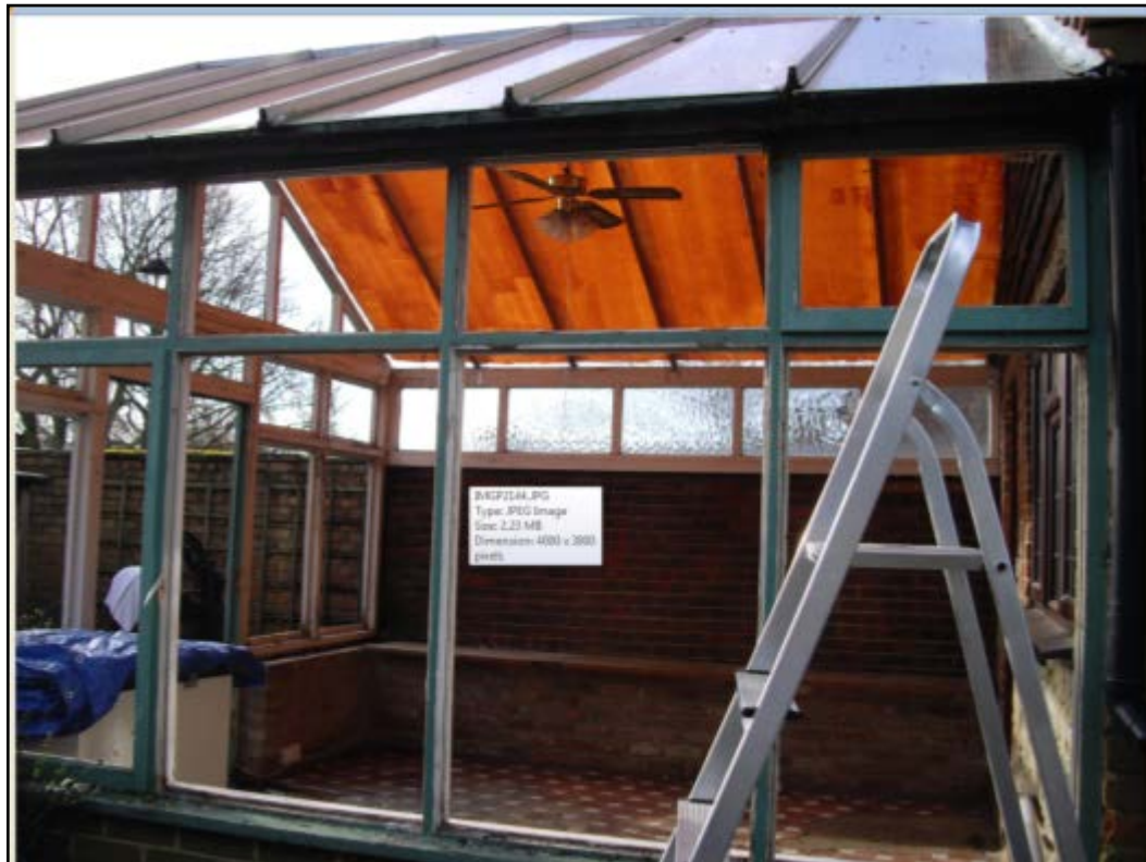
Figure 8. Picture of building/conservatory prior to rebuild works showing the high level windows on the side (NW) elevation facing the neighbour.
